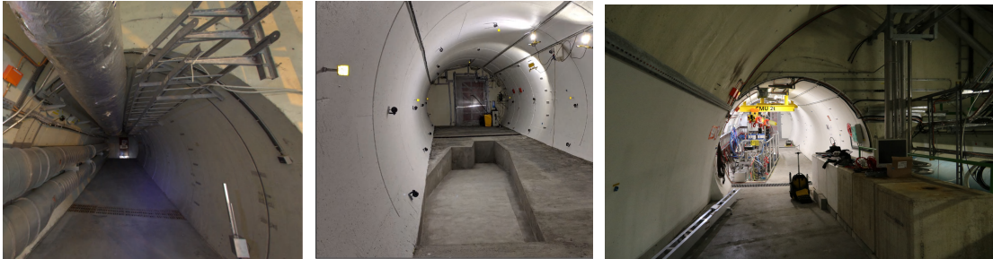
(a) Before FASER work in the TI12 tunnel. [8] (b) After TI12 cleared out and the trench finished. [8] (c) Current layout of FASER, during YETS 2023-24.
