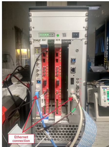
Figure 4.9: From left to right : the crate controller, the two digitizers and the TLB.
